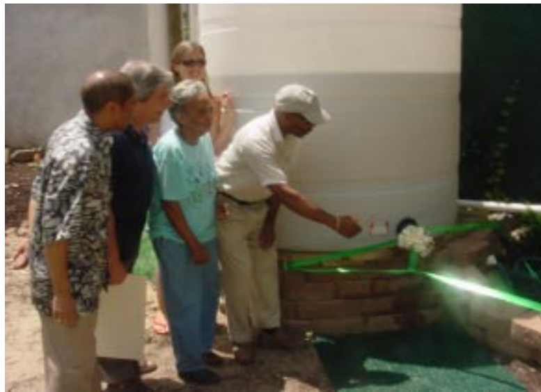
Members of First Quincy Street Community Garden cut the ribbon on the giant 1,000 gallon capacity rainwater collection system.
